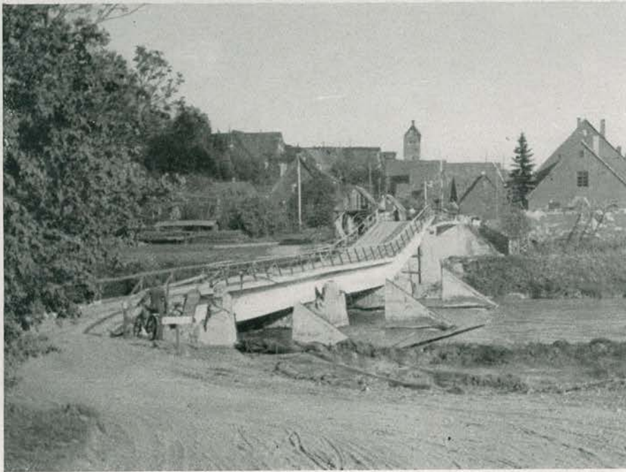
Another Danube bridge by 12th Armored Engineers. New structure is superimposed in the supports of the old bridge — south of Gundelfingen, Germany.
