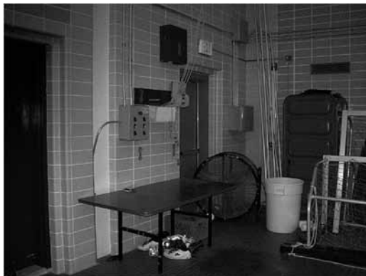
Figure 2 — Unorganized equipment blocking an exit.
