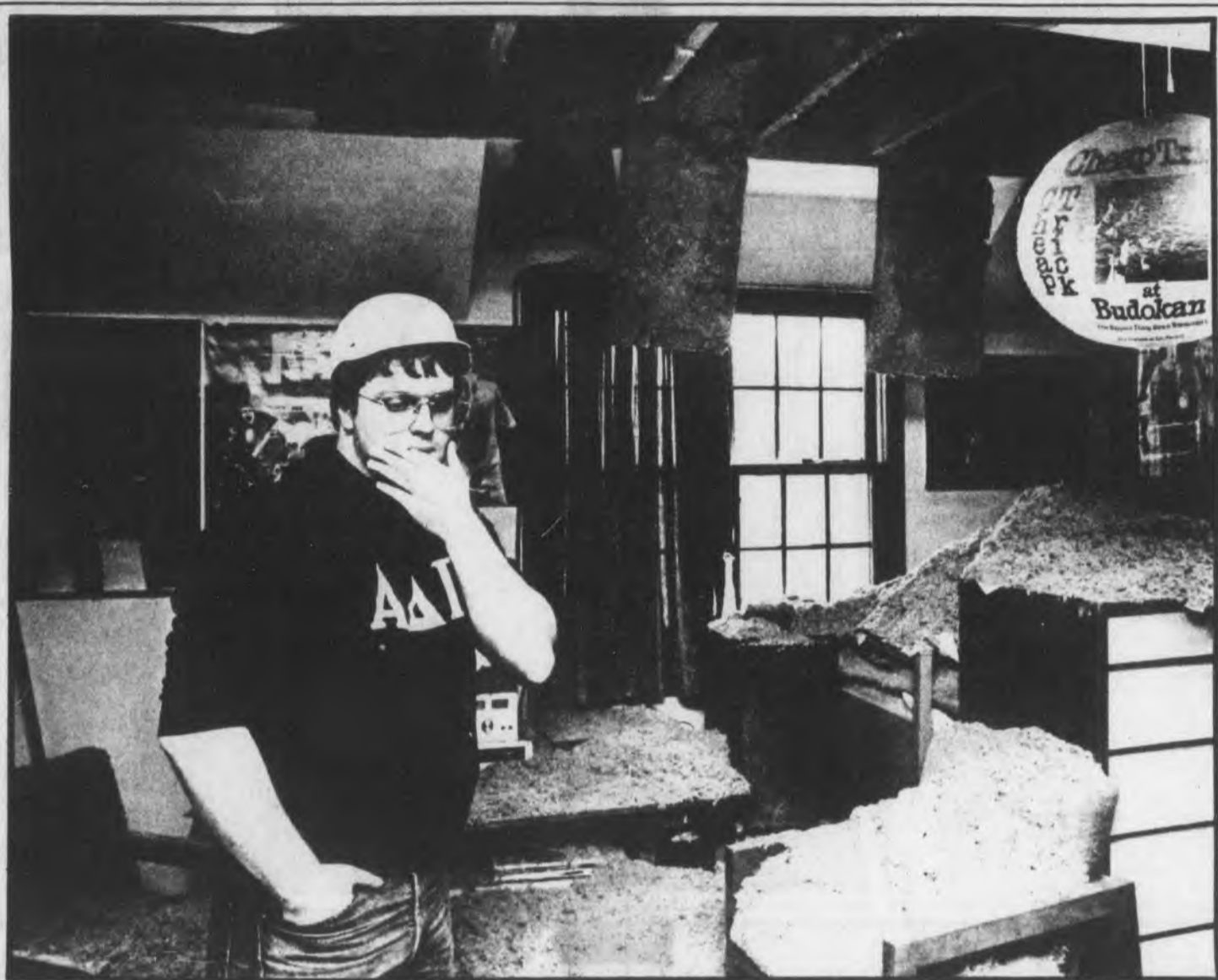
Brad Hanson, a junior visual communications technology major, surveys his damaged room.
