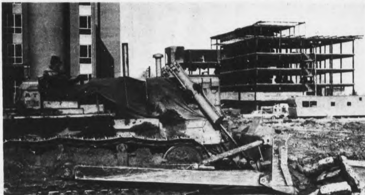
EXCAVATION BEGAN last week at the site of the new general science lecture building which is scheduled for completion in April, 1969.
