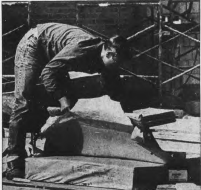
RAIN AND HIGH WINDS have not slowed construction on the University's new WBGU-TV station location behind the Delta Zeta social sorority house. A workman is shown cutting insulation material to be placed in the walls.
