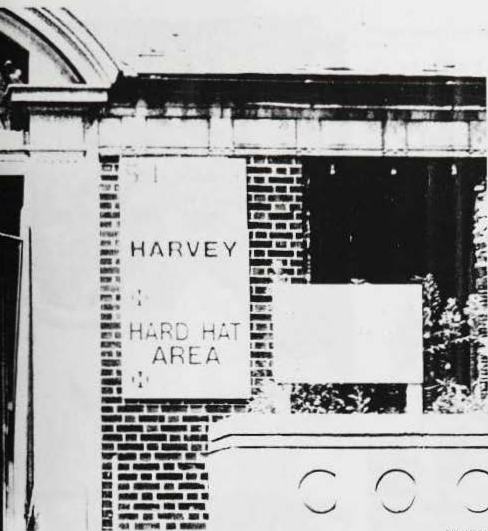
Early stages of the Cook Hall renovation required a hard hat for those in the area.
