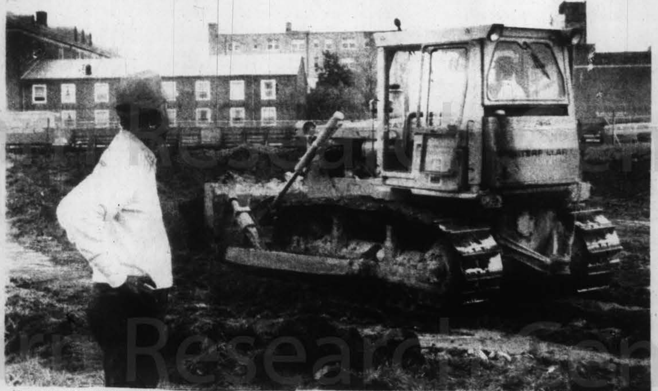
Head Track Coach Edward Moultrie observes a bulldozer excavating Howard Stadium on Monday.
