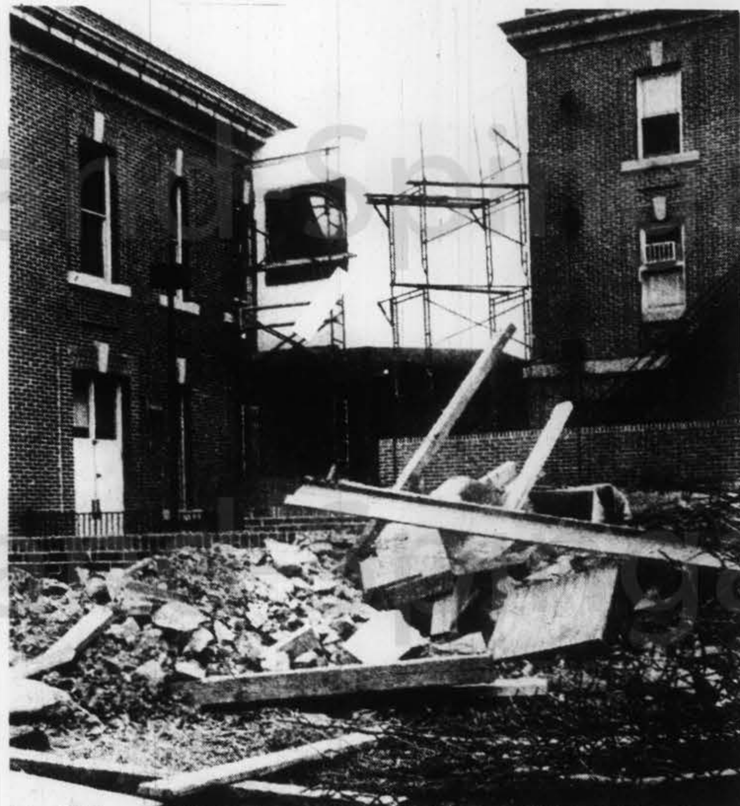
The construction site of the new Communications studio Hilltop Photo- Tad Perry
