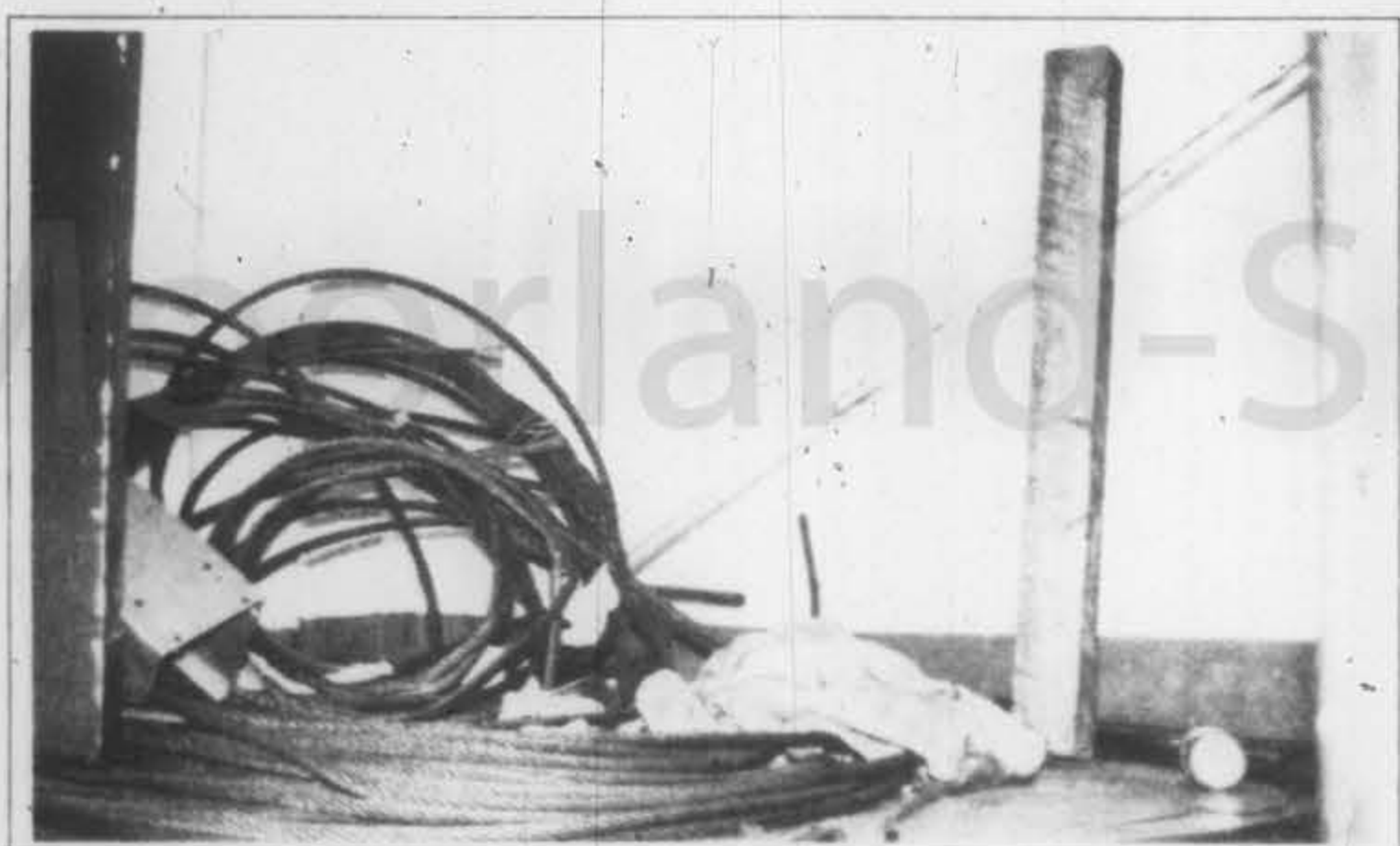
(Top right) The new motor and cables (above) will replace old equipment that was under scrutiny by dorm officials.
