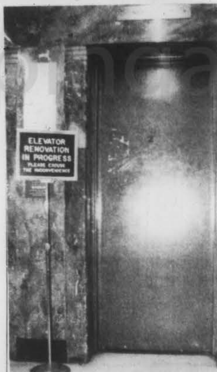
photos by Frank Byrd Elevators are off limits to students during the repairs.
