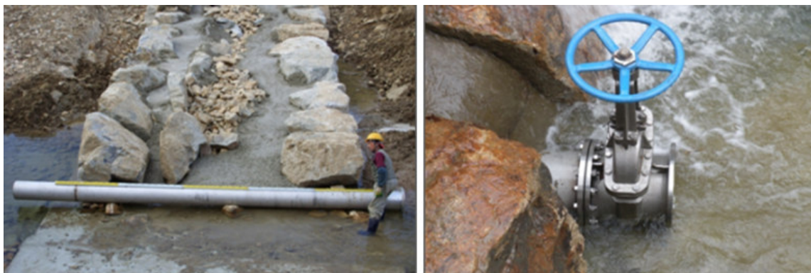
Figure 3. Improved drainage practices (water pipe \Phi 100\text{mm} \Rightarrow replaced by \Phi 300\text{mm} at the base area)
