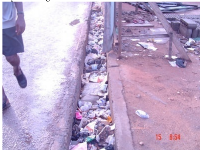
Figure 7: A gutter engulfed with solid waste.
