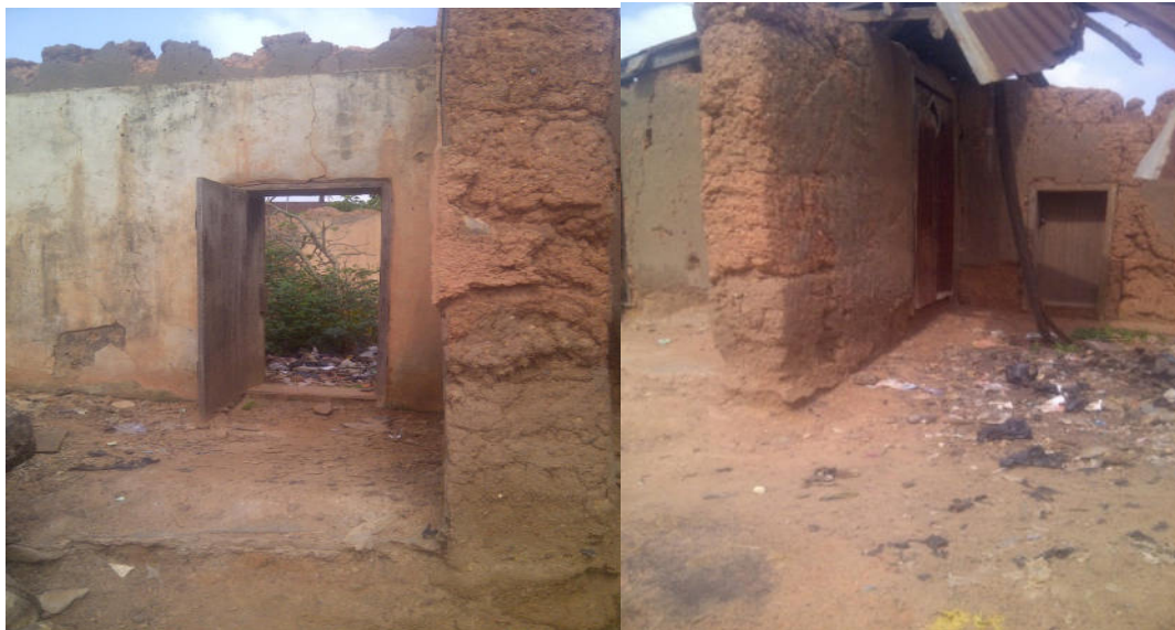
Plate 4: Dilapidated and Deteriorated Abandoned Structures in Oke-oyi Area.
