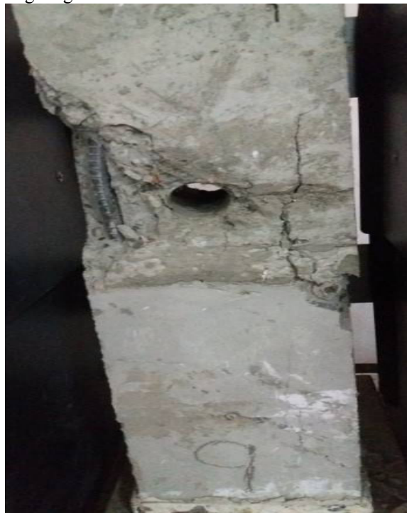
Failure mode of column, Fig # 02.
