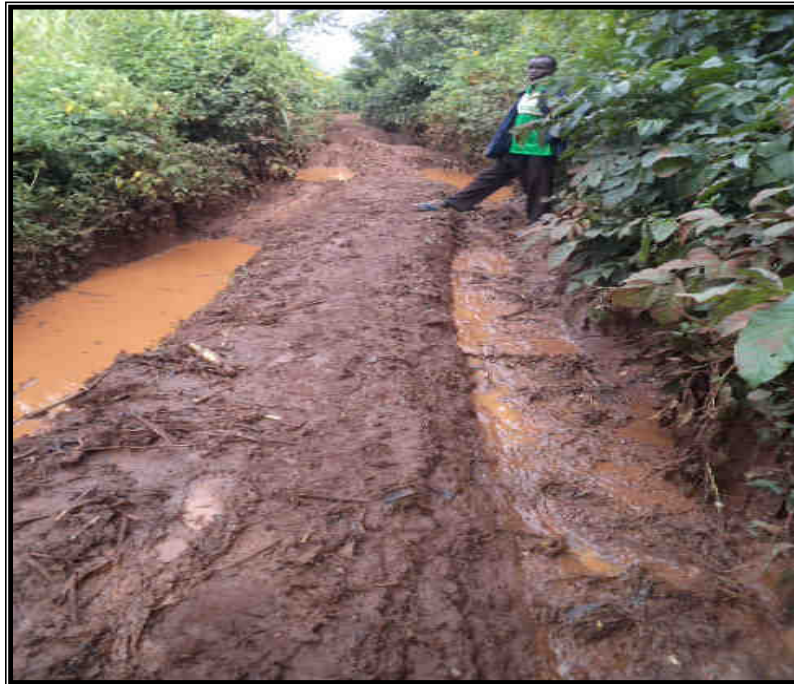
Plate 15: A picture taken by the researcher, in August 2012, of a section of a feeder road in Kivaywa in a bad state.
