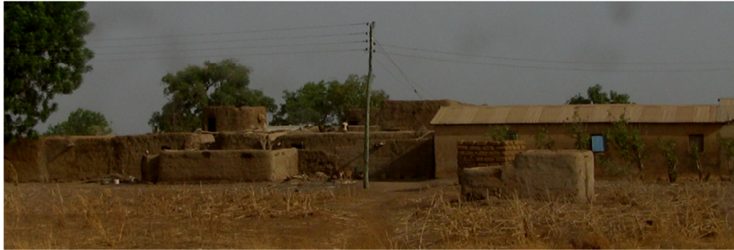
Figure 7: Present condition of the Dagara House with introduction of 'modern' metallic roofing material (photo: field survey, 2013)
