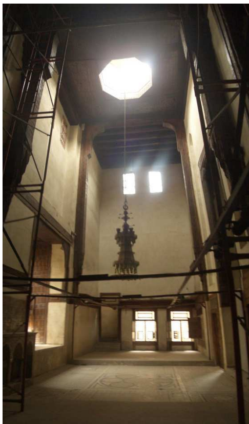
Figure 14: Reception Hall " Qa'a " of Zeinab Khatoun House. Source: survey by Abdel Gelil Mohamed, Nermine.
