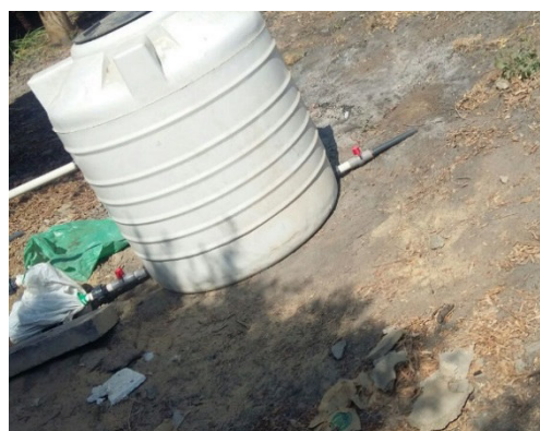
Figure 2: The settling tank
