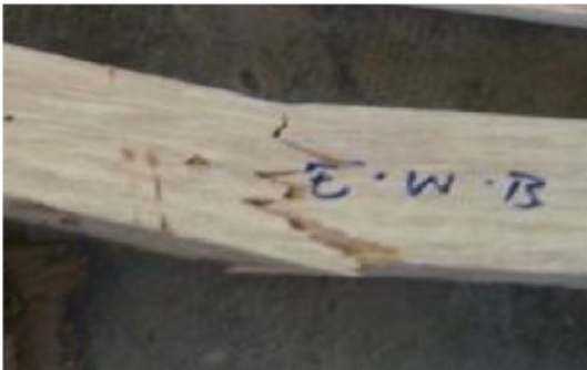
Plate 4: Bending failure in glulam
