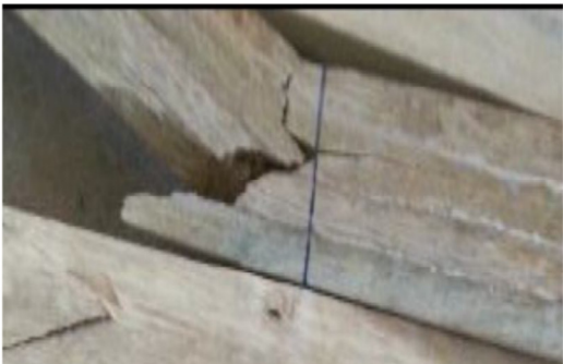
Plate 3: Bending failure in solid beam
