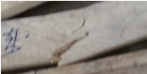
Plate 5: Bending failure in solid beam
