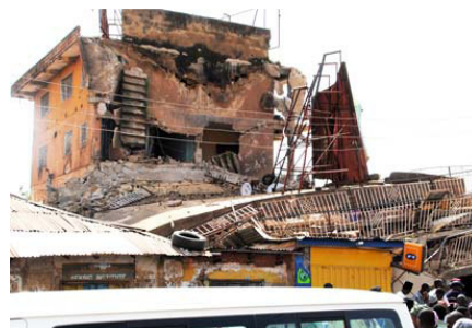
Figure 7: Collapse of Multi Storey Building in Kaduna.
