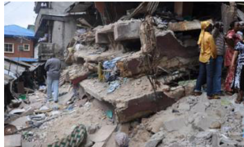
Figure 4: Collapse of Multi Storey Building in Umuahia, Abia, State, Nigeria
