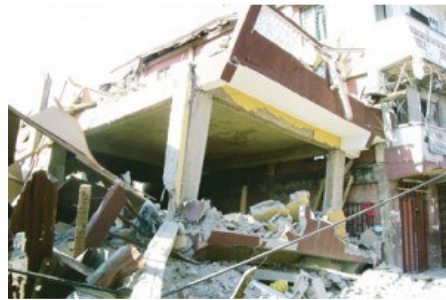
Figure 6: Collapse of One Storey Building in Kano.
