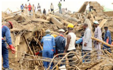
Figure 9: Collapse of Two Storey Building in Dutse, Abuja, Nigeria
