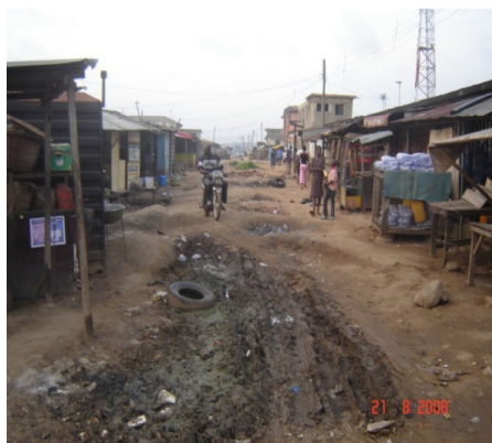
PLATE 1 Deplorable Condition of the Road
