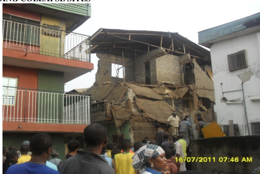
Figure 3 Collapse site at 20 Doyin Omololu Street Lagos State, Nigeria.
