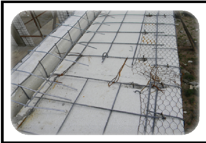
Figure 4: The top of the EPS fascia is connected to the EPS wall panel with binding wire and covered with L-shaped splice mesh for strength, rigidity and continuous reinforcement. A Bungalow at Mbora Mount Pleasant Estate Abuja Source: Authors' Survey 2010
