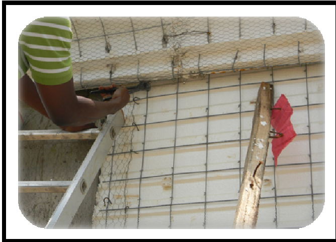
Figure 3: The bottom of the EPS fascia is connected to the EPS wall panel with binding wire for strength, rigidity and continuous reinforcement. A Bungalow at Mbora Mount Pleasant Estate Abuja Source: Authors' Survey 2010
