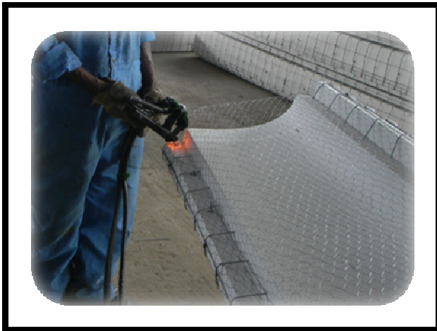
Figure 1: EPS Fascia reinforced with wire mesh and covered with chicken mesh during production at CIBPL Abuja Source: Authors’ Survey 2010
