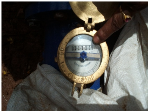
Figure 2. Bulk Flow Meter at Lingarajnagar, Hubli
