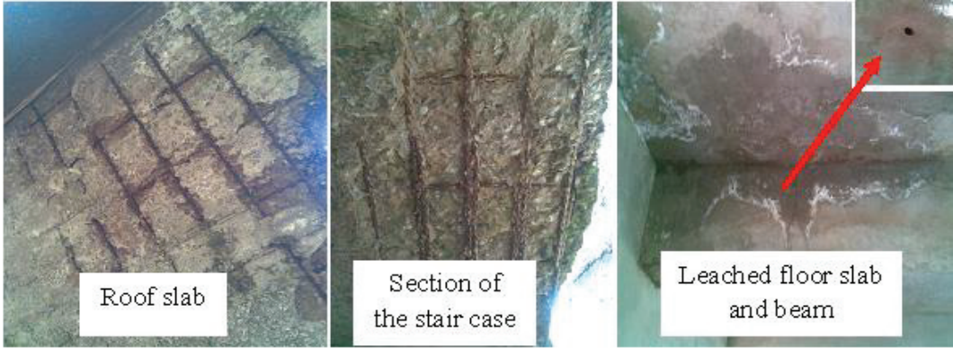
Figure 5: Rebar corrosion of stalled building at Kapsuya Secondary (Eldoret)
