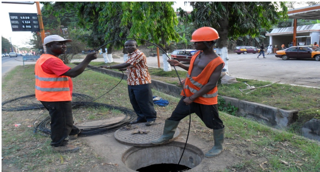
Picture 3: Fiber cable being pulled by Vodafone staff as it arrives at a junction
