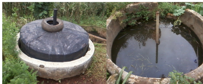
Figure 5.2.1 Common problems with biogas plants in Western Kenya; low biogas production/gas leakage (left) and structural collapse (right)
