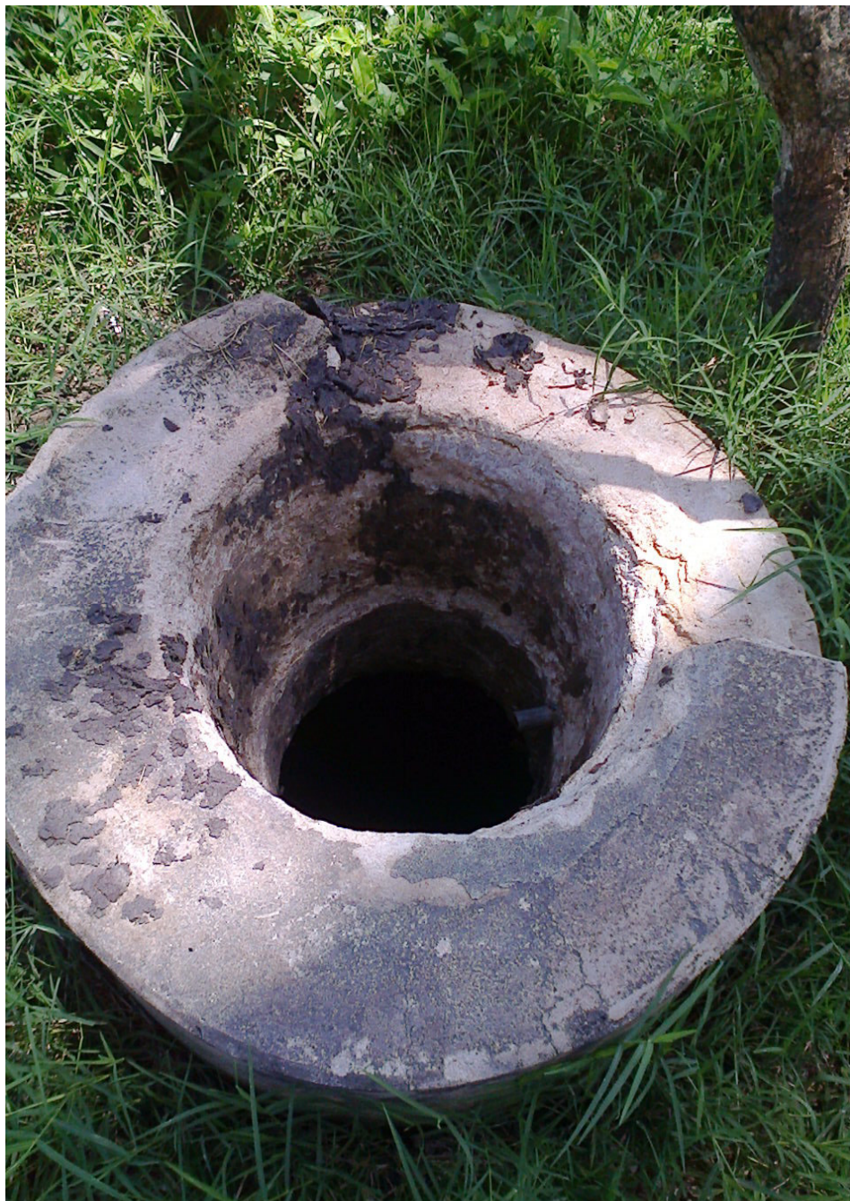
Figure 4: Abandoned biogas plant due to lack of technical services (Source: Field study done by author 2014)
