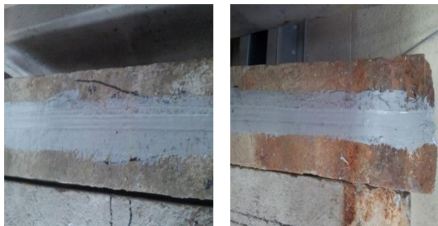
a. A1T Control.Beam b. A1CL3 Corroded. Beam
