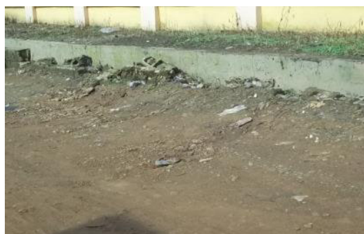
Plate 7: A Badly damaged Drain at Dele Johnson Street Due to Improper Construction
