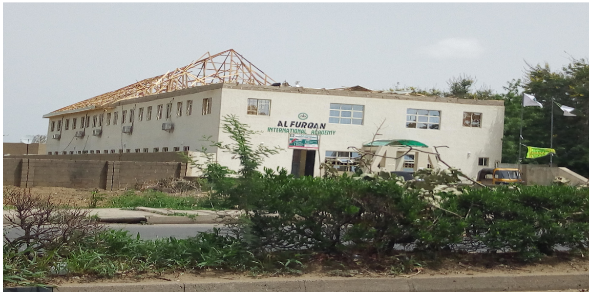
Plate 1: Uprooted roof of Alfurqan International Academy along Abubakar Tafawa Balewa Road, Bauchi Source: Researchers' Field Observations, 2018
