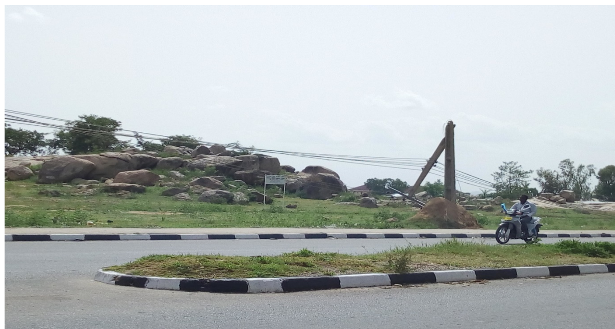
Plate 2: Damaged street infrastructure along Bauchi-Jos Expressway. Source: Researchers' Field Observations, 2018
