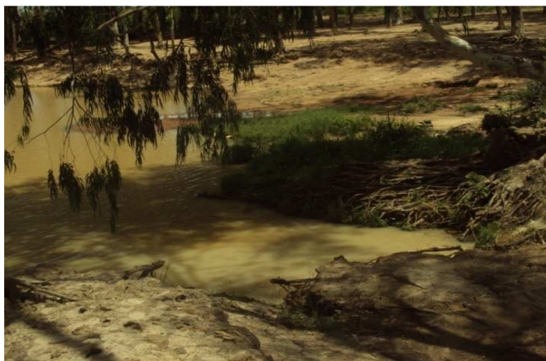
Fig. 2. A portion of eroded reservoir embankment showing shape irregularities
