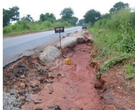
Plate 2 : Pavement conditions at some Locations on Irrua - Auchu road
