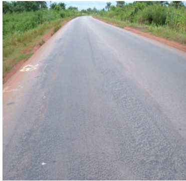
(a) BLEEDING AT CH.27+000
