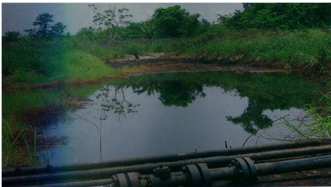
Fig. 6: Spill caused by removal of Bolts and Knots from Flow Lines with Free Oil February, 2005.
