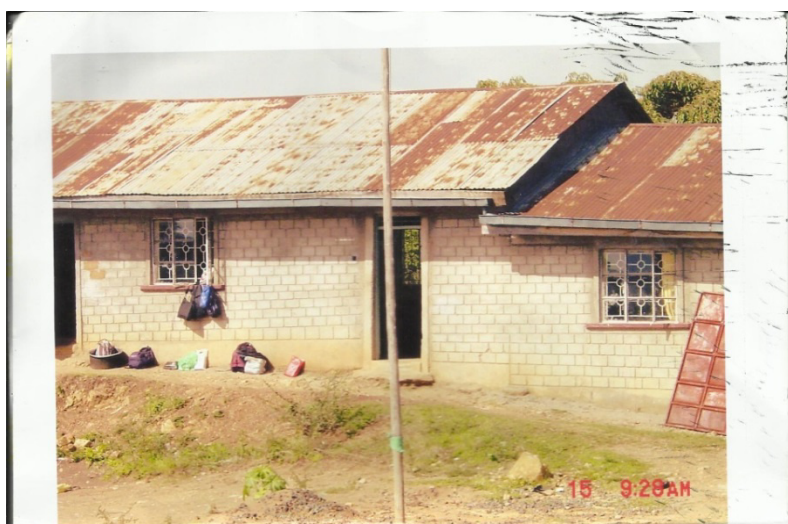
Figure 2: The condition of doors as entrance to classrooms
