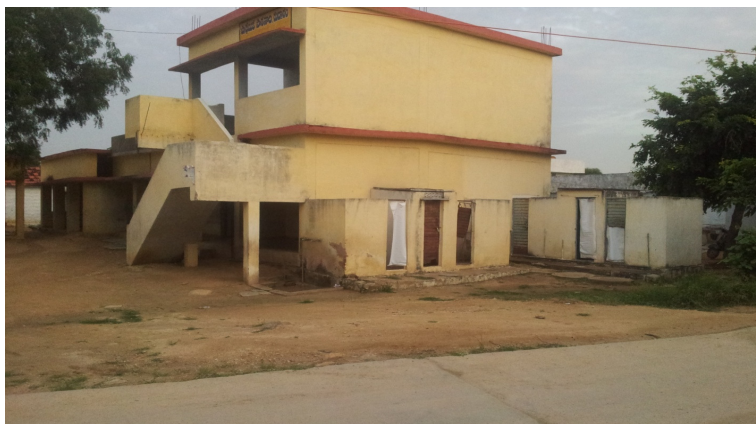
The Zilla Parishad Primary School building without a compound wall and unusable toilets.
