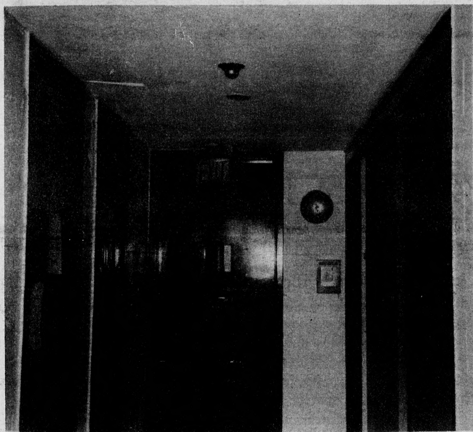
Non-operational ninth floor fire alarm bell in Bohn Hall
