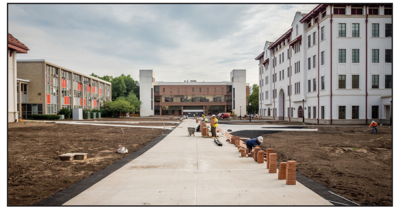
Construction is underway on a promenade running between CELS and Mallory and Shmitt Halls. Photo Courtesy of Mike Peters.
