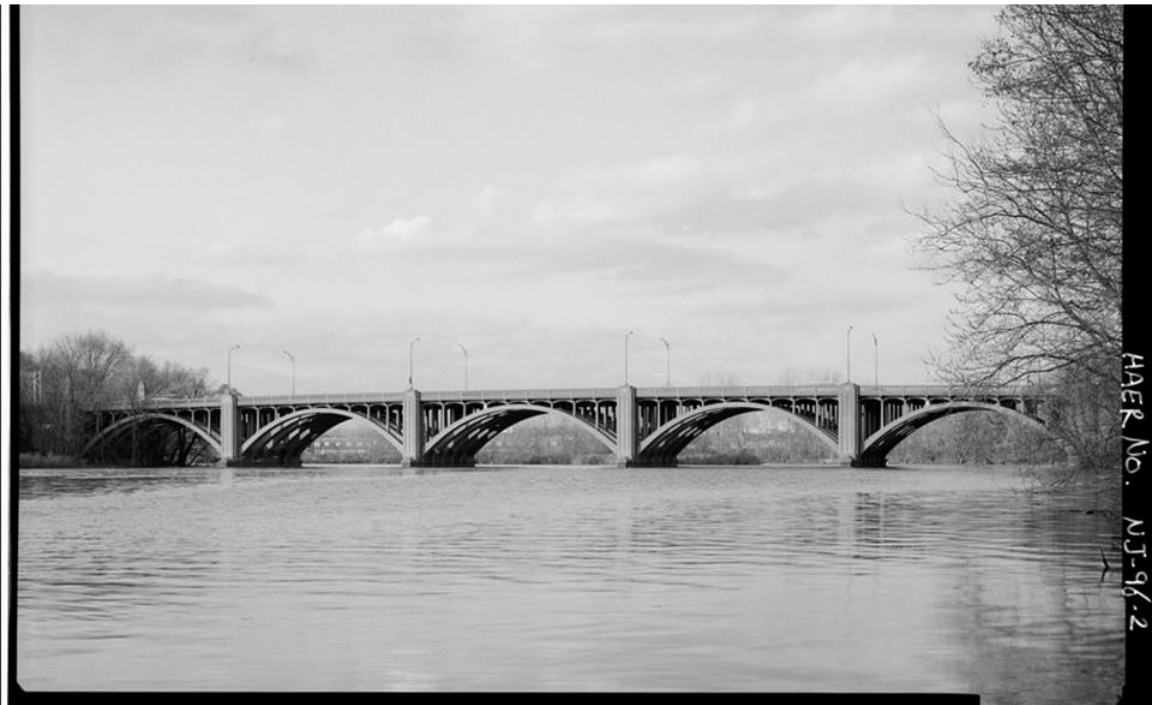
Figure 3-2. Looking Upstream at the Route 46 Highway Bridge. Due to the significance of its concrete arch construction, the bridge was placed on the National Register of Historic Places in 1991. (Library of Congress)
