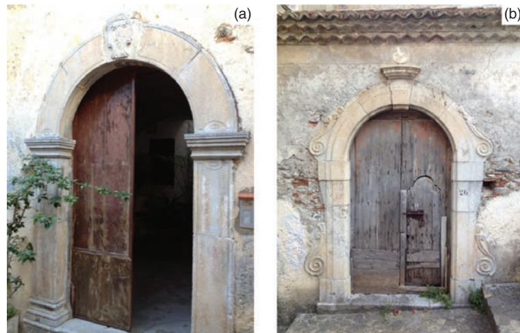
FIGURE 11. Examples of portals realized with Grisolia stone and affected by slight decay forms.
