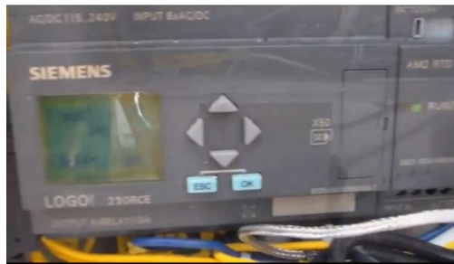
Figura IV.40. Logo 230 RCE Tablero de Control 50
