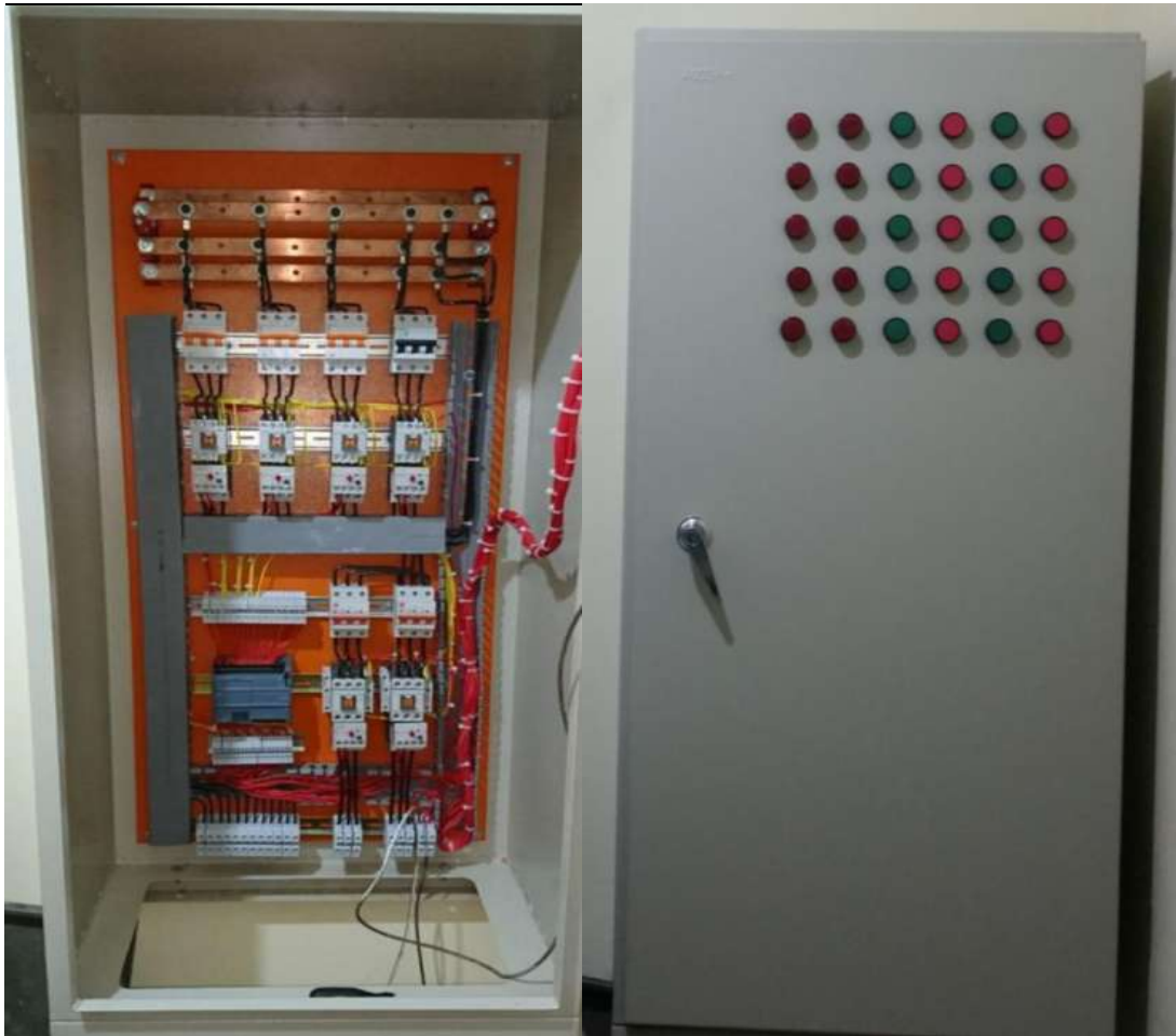
Figura 42-2: Tablero de control instalado
