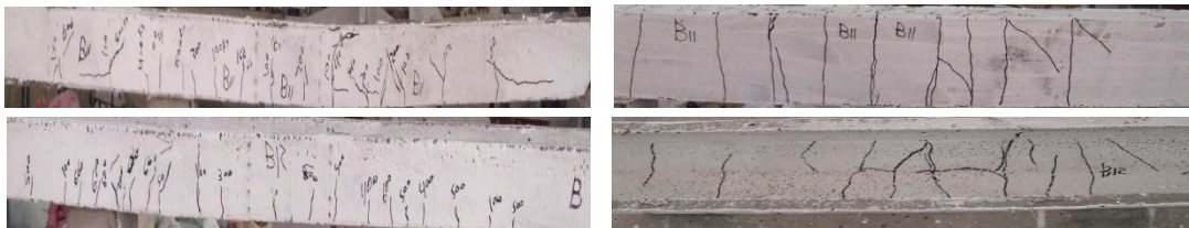
Crack Pattern from side of the beam
