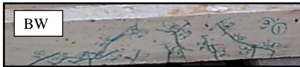
Figure 27. Crack Pattern for beam (BW) after 15 days of Corrosion Acceleration
