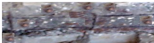
Figure 23. Corroded beam after 15 days of Corrosion Acceleration
