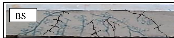
Figure 32. Crack Pattern for beam (BS) after 60 days of Corrosion Acceleration
