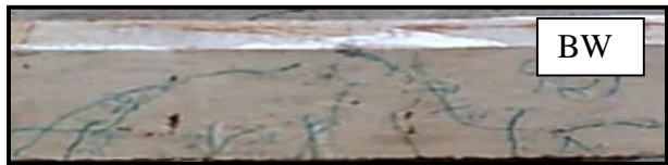
Figure 24. Crack Pattern for beam (BW) after 30 days of Corrosion Acceleration
