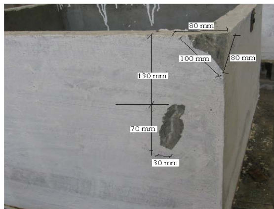
Figure 4. Damage Ferrocement Tank.
