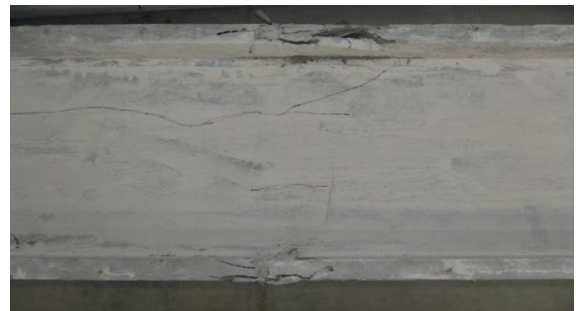
Crack pattern of S9
