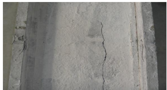
Crack pattern of S10
