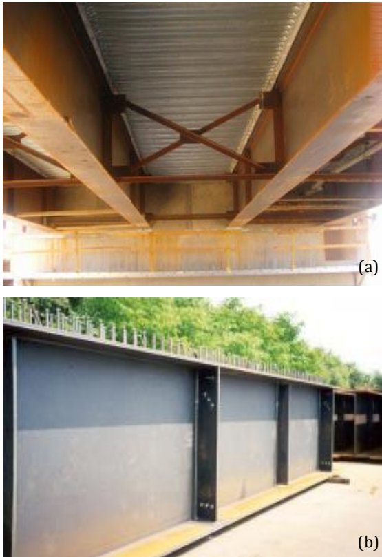
Fig. 1. (a) Typical steel-concrete composite bridge, (b) Steel girder with stud shear connectors.
