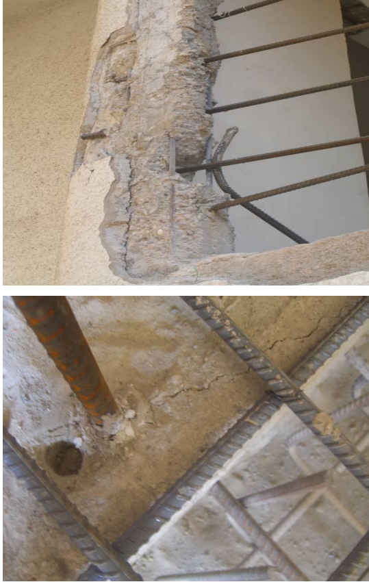
Fig. 1. Concrete quality and anchor workmanship in some strengthened structures.
