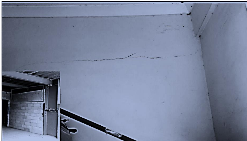
Fig. 4. Steel structure under construction and cracks between infill walls and steel frames.
