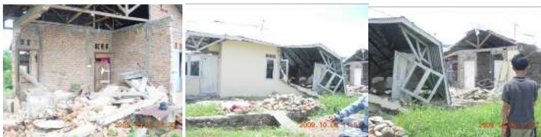
Figure 1. Condition of Masonry Houses after earthquake
