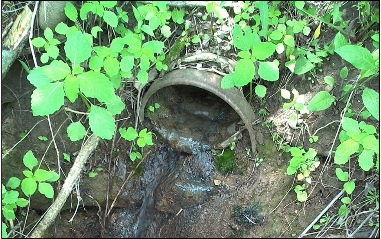
Figure 60. Drainage pipe outflow that was used to sample water from Stream B until 10/20/15.
